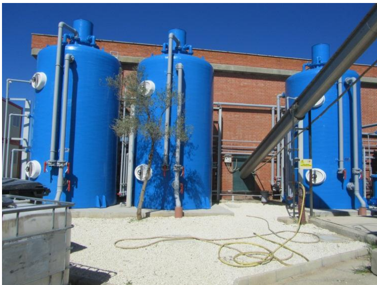
• UASB digesters at Chiclana
